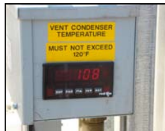
Temperature indicator from extreme-duty vent condenser in operation.
